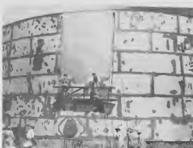
PAINT CREWS test the new DeVilbiss paint spray on a tank. Teams of three painters each tried out the spray.
